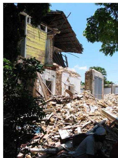
Centre d'Art collapsed building and site, Port-au-Prince. Photograph by Stephanie Hornbeck.
